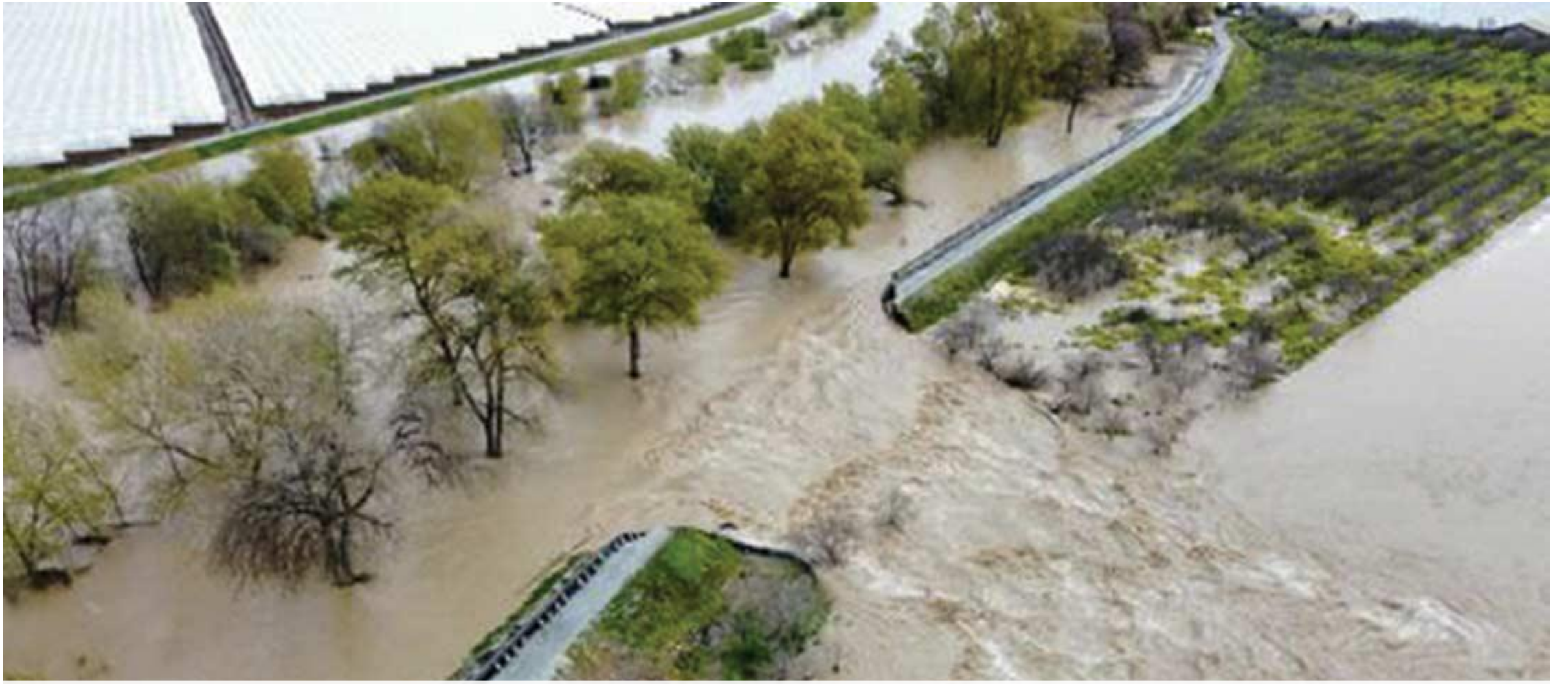
Pajaro River Levee Breach, March 2023
